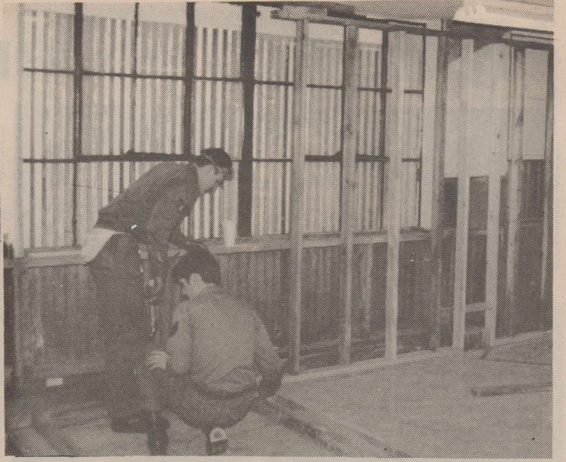
SSgts. Steven Broom and Don Elson from TOT section build a wall in a classroom of Hanger 70.
