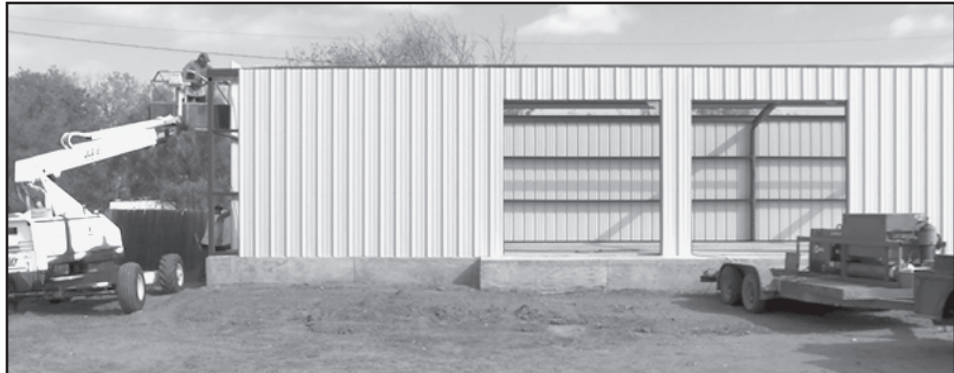
NEW DISTRIBUTION LOCATION —A new 30x60 metal building is being built on Hwy. 380 East in Haskell across from East Side Baptist Church to house a distribution center for Frito-Lay. T's Welding is the contractor. The building is owned by Ben McGee.
