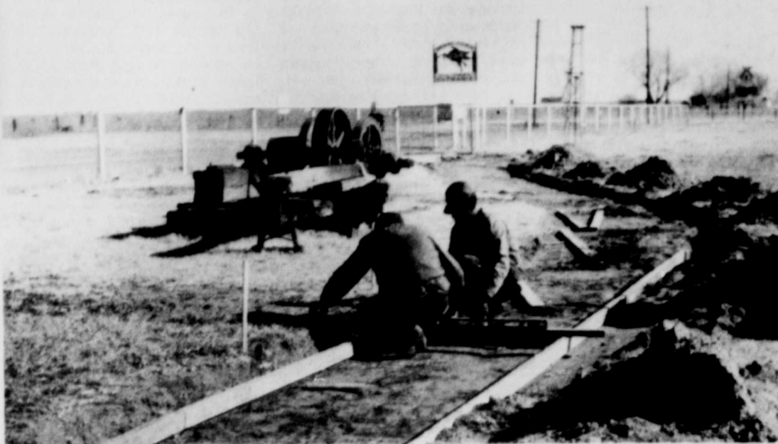
Burkburnett City workers J.D. Mullins and Bill Arron lay sidewalk for the Boomtown City Oil Park.
