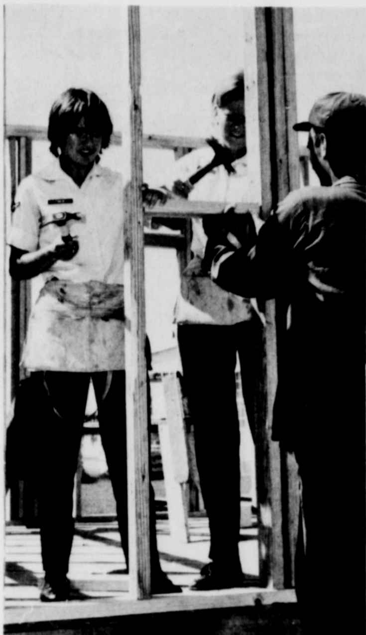
BUILDING STRUCTURE-- Airman Kim Farlin and Airman Basic Patty Willis work on a structure in their carpentry course at Sheppard's School of Applied Aerospace Sciences. Working with them is Airman Basic Charles A. Holden. Airman Farlin and Willis were the first enlisted women to enter the carpentry career field in the Air Force. (OFFICIAL USAF PHOTO BY AIRMAN FIRST CLASS LARRY ORR)
