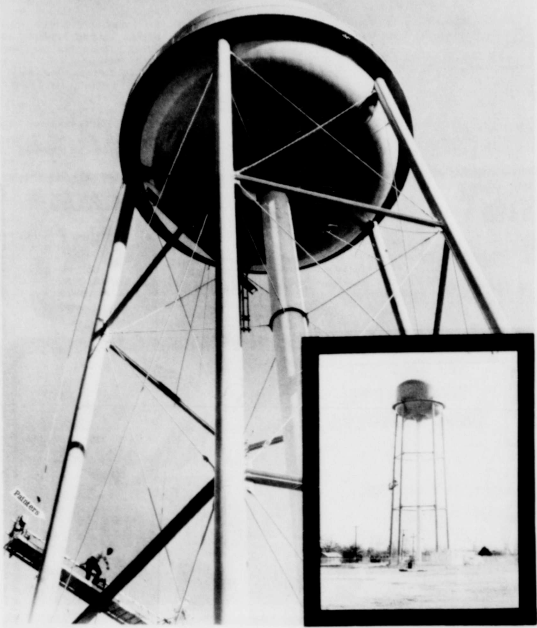
PAINTING THE TOWN ORANGE--Painters were contracted recently to paint the two water towers in Burk Burnett orange to match the school colors. Also on the towers will be black lettering. On one tower there will be a painting of a bulldog with lettering which says, "Burk Burnett Bulldogs". The other
