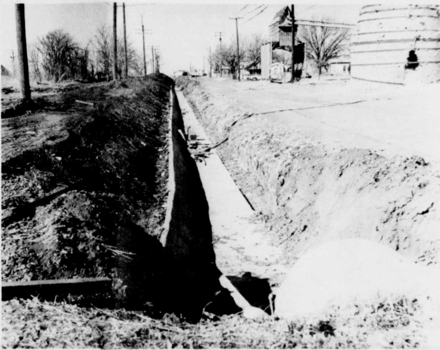
DRAINAGE DITCH--A 1,400 ft. concrete-lined drainage ditch running north on 4th Street was recently built. This ditch drains all of the downtown area of Burk Burnett. Shown in the photo is
