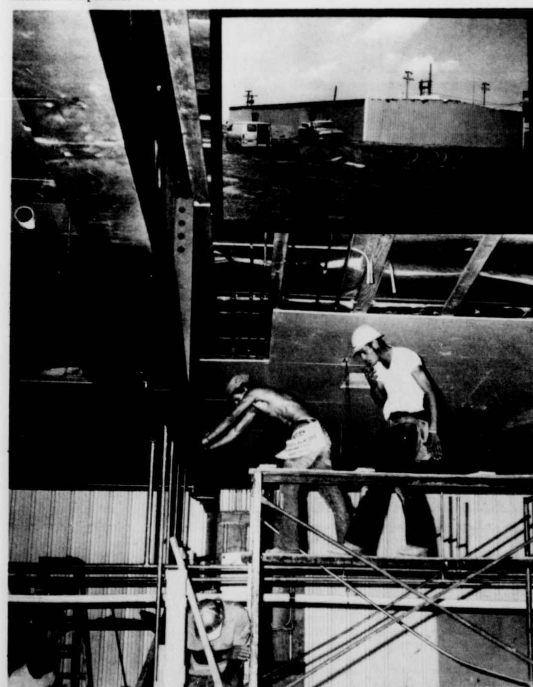
PUTTING A FIELDHOUSE TOGETHER--Workmen have been steadily working at completing the new 6,000 square foot fieldhouse which is located south of the high school football stadium. Pictured is a scene from the inside showing ceiling and wall
