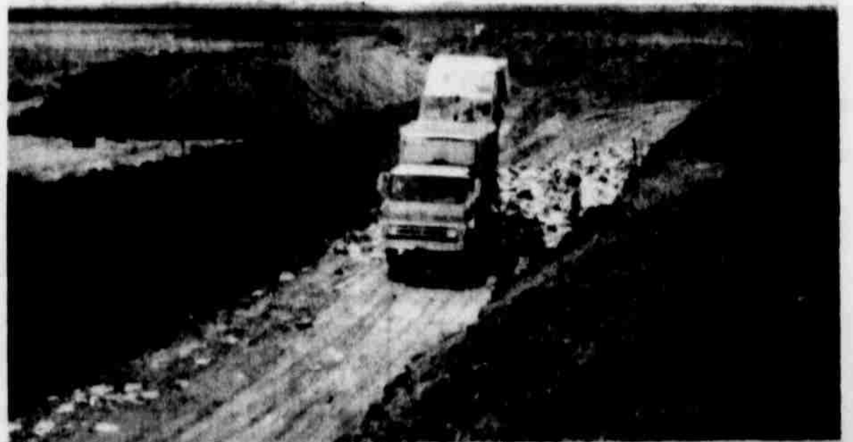
NEW LANDFILL PROGRAM at the City Dump is now in full swing. The trench, 300 feet long, 30 feet wide, and 10 feet deep, was built so that the City would meet recent State sanitation requirements. A second trench for brush and trees is now complete. The trenches should last from six months to one year.
