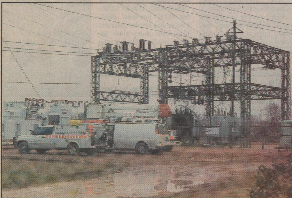
A mobile substation on a flatbed trailer was moved to the Winters substation by AEP Texas this week after a power outage Thursday night and Friday morning. The mobile substation will serve the community for about a month until permanent repairs can be made.
