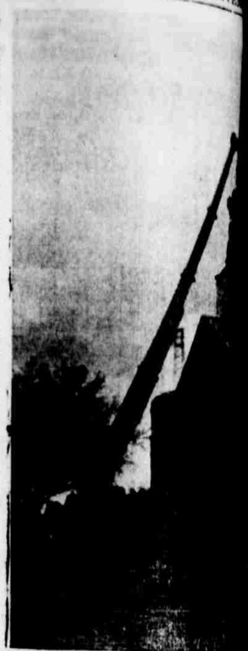
MEMBERS OF THE Haskell First Baptist Church are proud of the new steeple which was mounted on a 39 foot structure made of fiberglass and wood.
