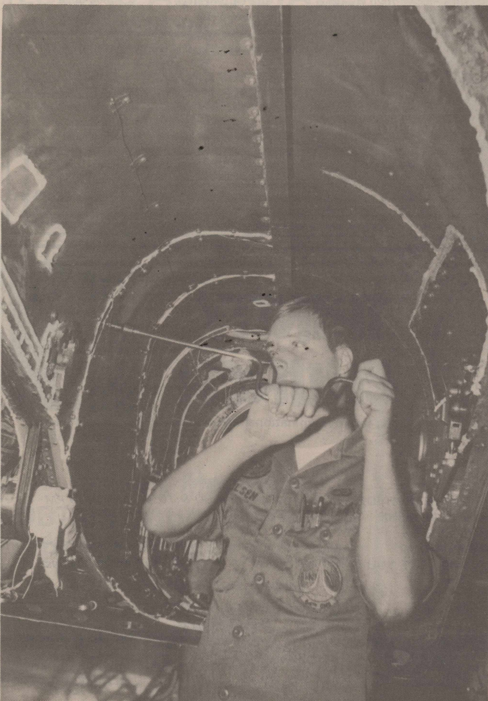
Airman First Class Robert Carlsen installs a firewall panel in a T-38. (USAF photos)
