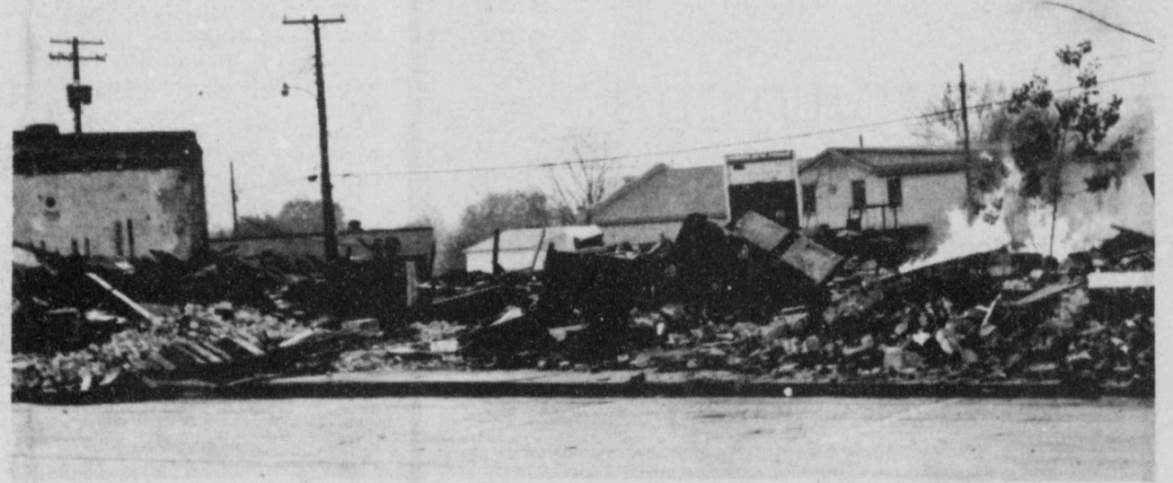
CLEANING UP-Workers are in the process of cleaning up the debris on Main Street in Bogata
