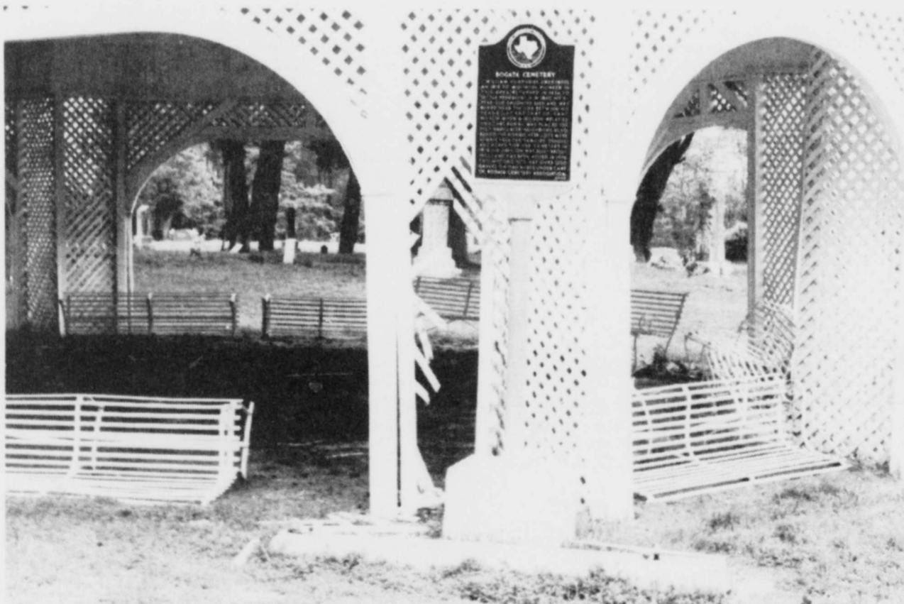
VANDALISM-Bogata Cemetery received damage to the pavilion and benches recently. A large hole
