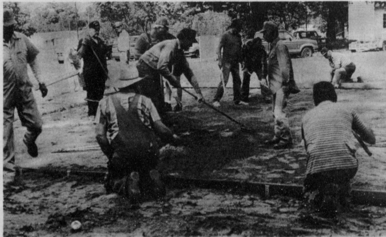
GETTING READY- This busy group of Rosalie men are getting the ground ready for the concrete to be poured for the pavilion of their new community center. (Photo by Judy Screws)
