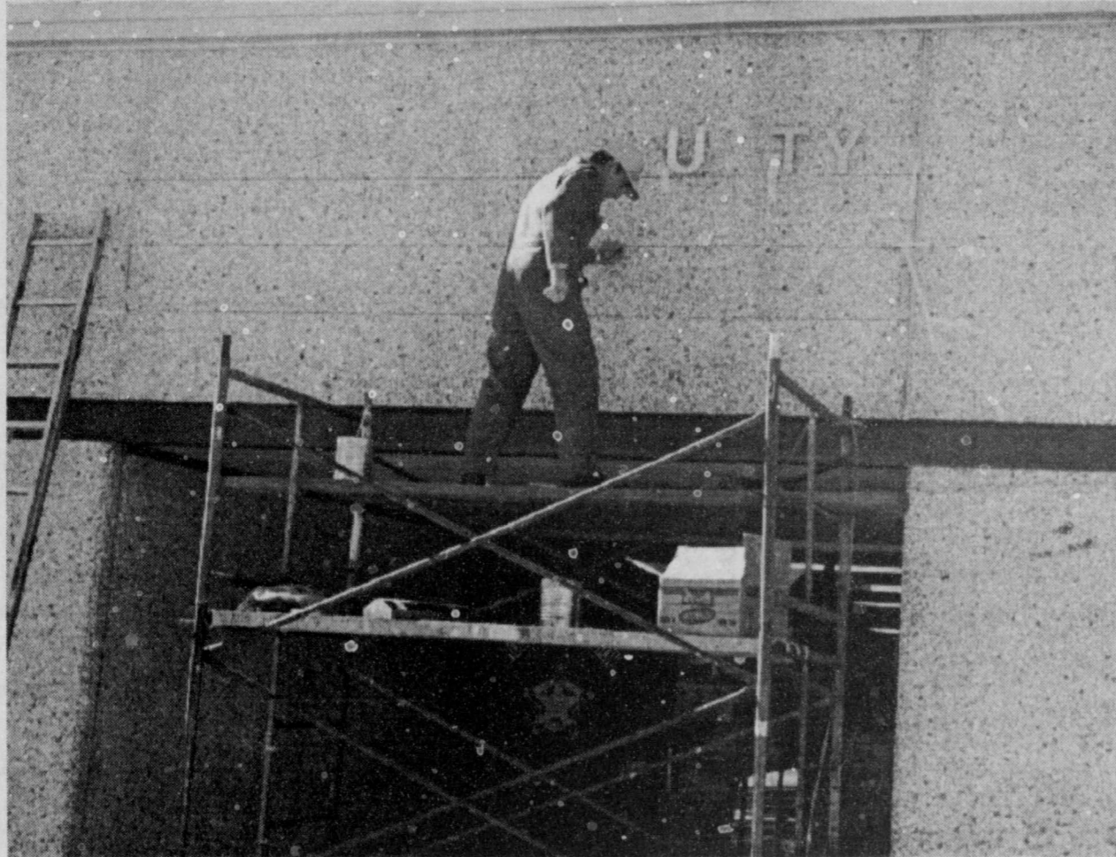
LETTERS for the Red River County Jail and Sheriff's Officer were being installed by workmen last Monday. The new 82 bed facility is almost complete and Open House was held last Saturday, Nov. 26. (Staff Photo by Thomas Nichols)
