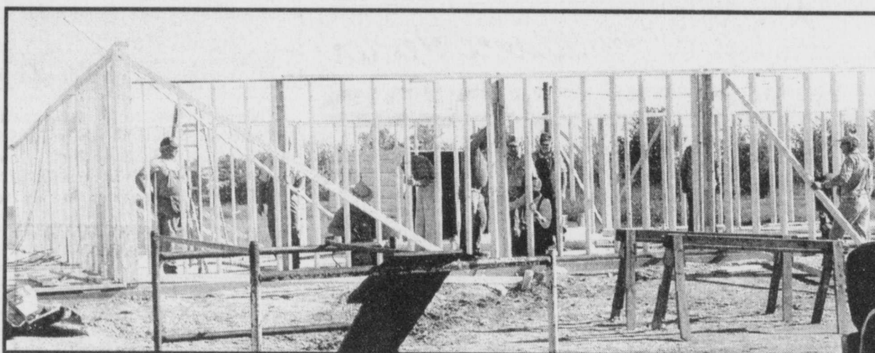
The construction crew began work on Bogata Missionary Baptist Church Monday, October 26. The labor on this new building is being furnished by Missionary Baptist Volunteers. (Staff Photo by Judy Screws)
