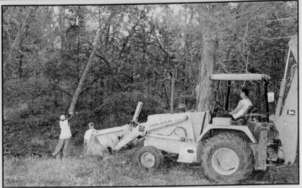
COMMUNITY WORK- Workers from the Red River County jail have been busy helping the city of Bogata clean dead trees out of the creek through Thomas Park. Many of the trees died last year as a result of drought conditions. The trees were restricting the flow of water as well as being an eye sore to Park users. Mayor Michael Garretson plans to use the jail inmates to do other work in the city in the coming weeks. (Staff photo by Thomas Nichols)
