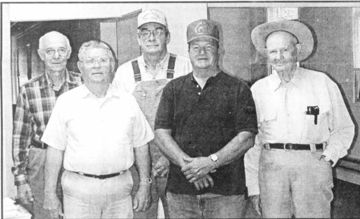
VOLUNTEERS-who have been busy removing walls and remodeling the Bogata Library/Museum in preparation of opening day are; A.D. Stephenson, Gaston Puckett, Neil Rozell, Carlton Stanley and W.T. Harbison. The men along with the help of many others have the building shaping up fast. (Staff Photo Nancy Brown)
