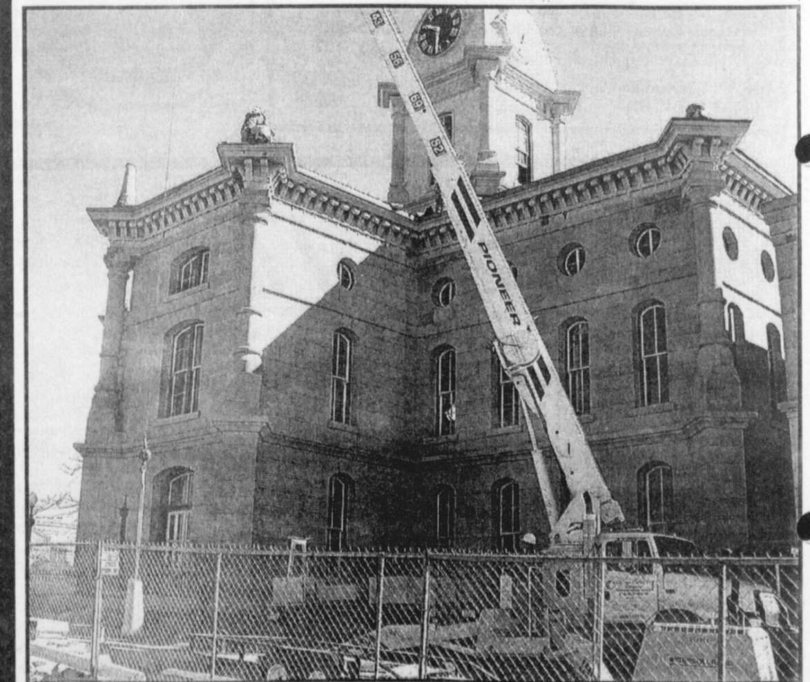
WORKERS are finishing up on the exterior of the Red River County Court House. The corners are being fitted with concrete turrets that weigh over a thousand pounds each. When complete, each corner will be over seven feet tall. (Staff Photo by Thomas Nichols)
