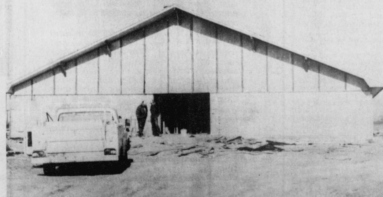
FIRST BAPTIST -the First Baptist Church of Deport, being constructed just east of the Deport
