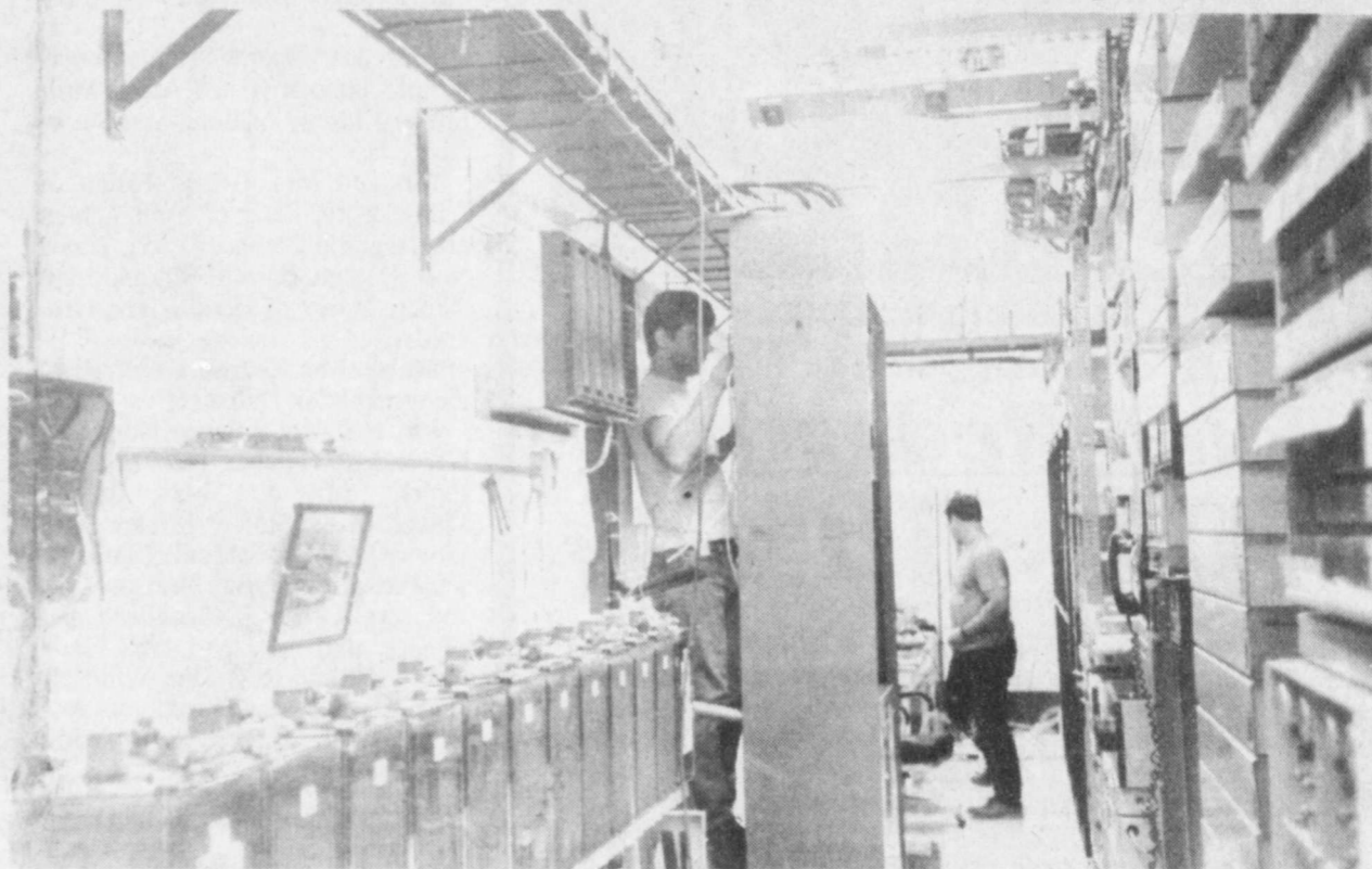
INSTALLATION-Workmen install a digital telephone system that allows speed dialing and speed calling at Blossom Telephone Company. The company is a privately owned company, owned by the Dorries family since 1950. (Staff Photo by Wendy Milford)
