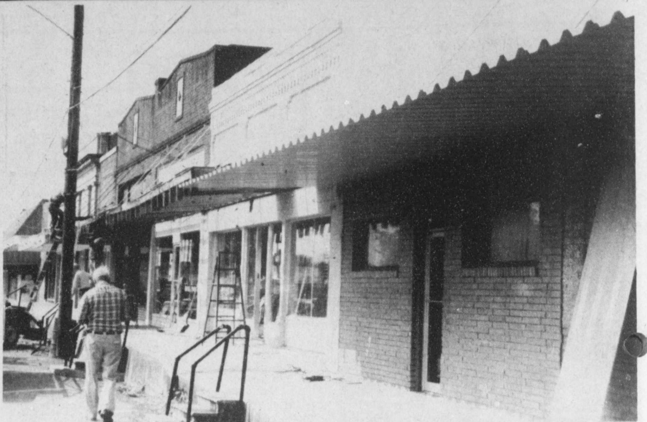
NEW LOOK-Dr. T.H. Glover's clinic, Deport Variety Store and City Drug received a facelift recently as Darden-Sparks Metal Construction put up new awnings. (Staff Photo)
