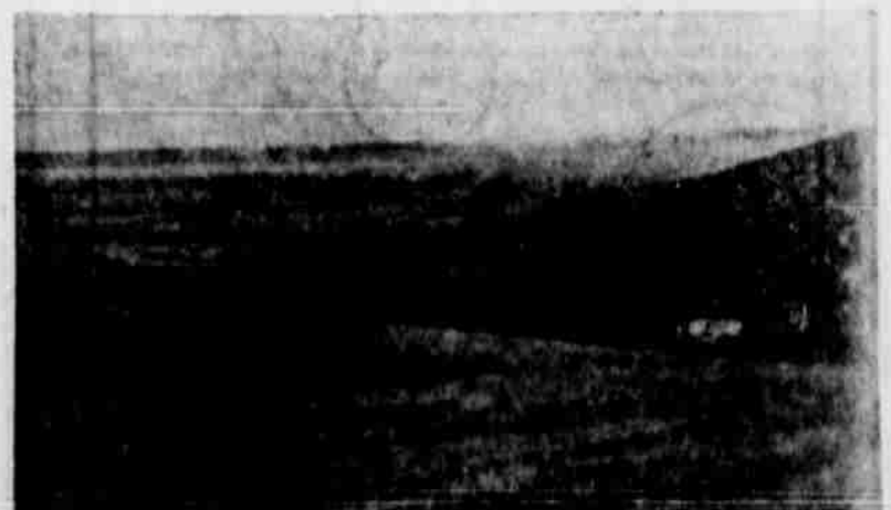
MILLER CREEK LAKE dam is in the final stages of completion, as this picture shows. Heavy equipment is now filling in the center portion of the dam, but elevation all the way across the dam is high enough that all spring rains will now be caught, and held, while the top of the dam is being completed.
