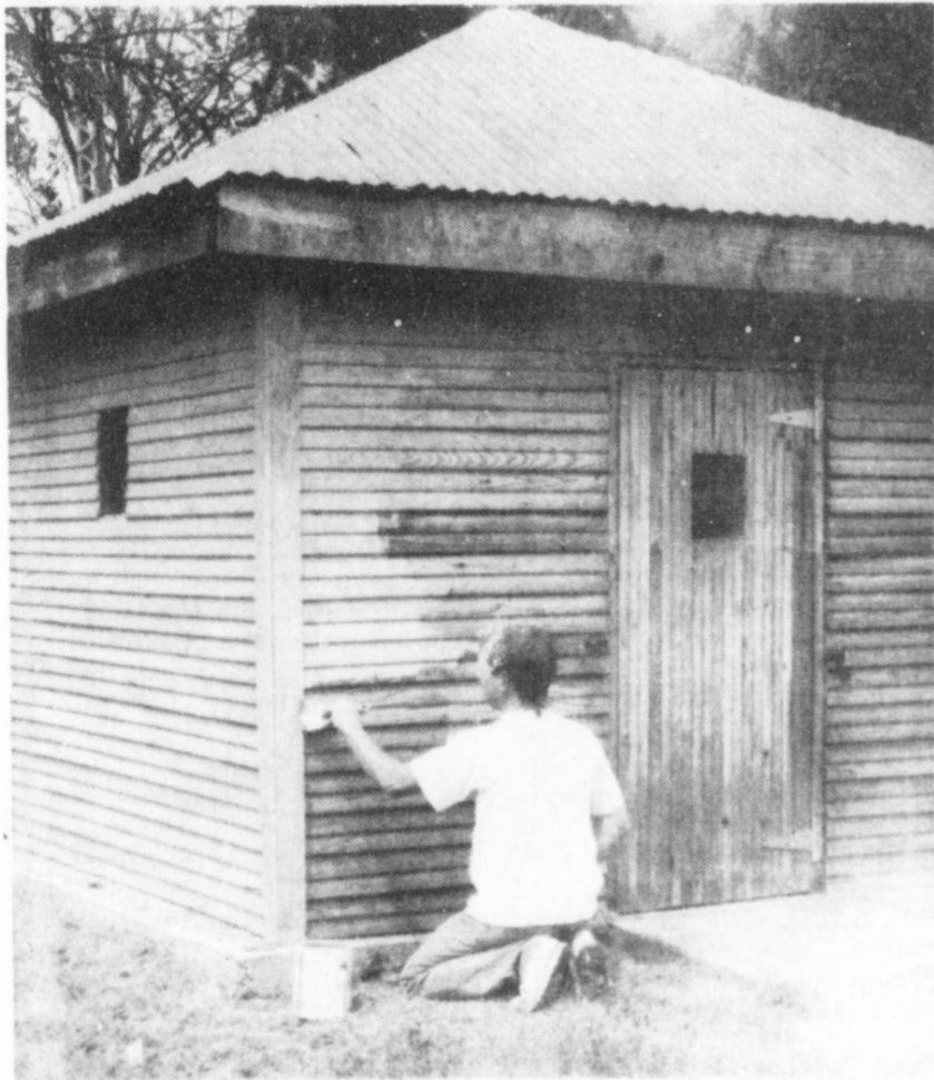
SPRUCING UP--Mike Francies donated materials and labor to water seal and stain the old
