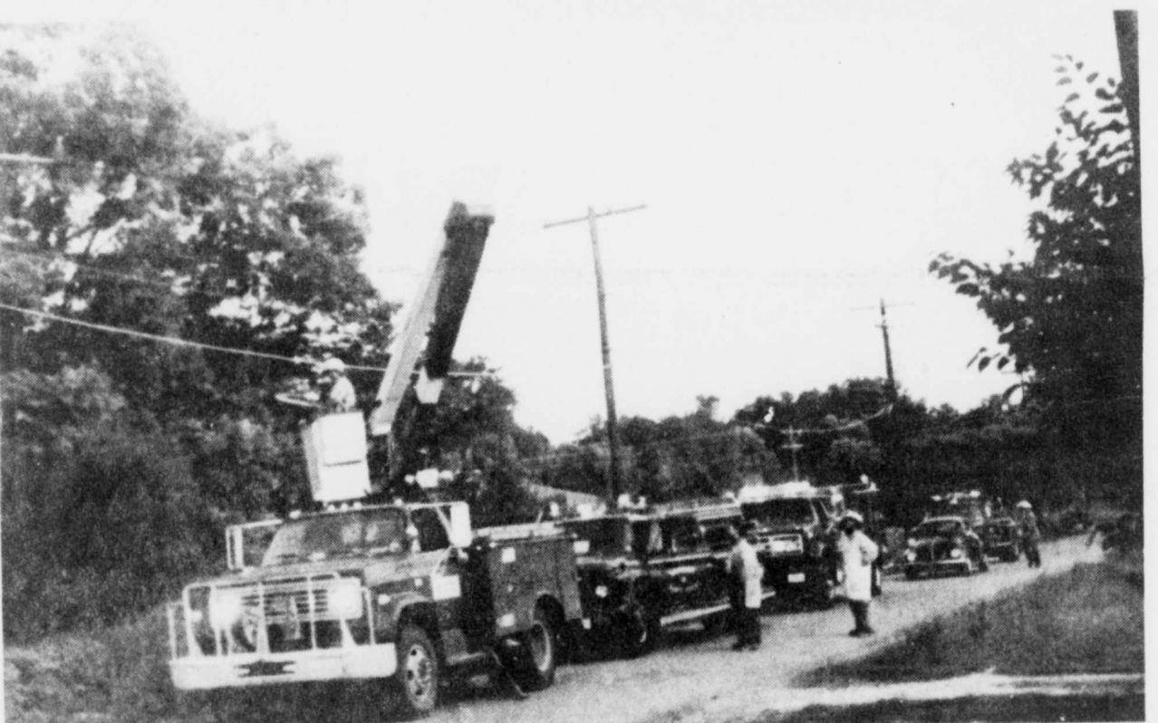
OUT!-There were power outages last Saturday afternoon, June 20 as a storm came through with high winds but no rains. A pole and transformer in a pasture behind Deport Nursing
