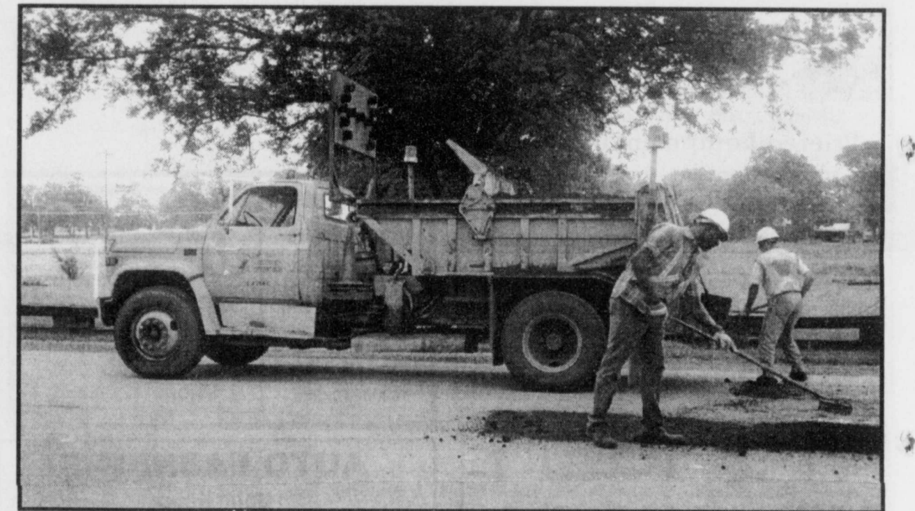
PATCHING-TxDOT employees were on Main Street in Deport this week patching some spots in the road. Cooler weather has made work like this and yard and garden work a pleasure recently. (Staff Photo by Liz Irwin)
