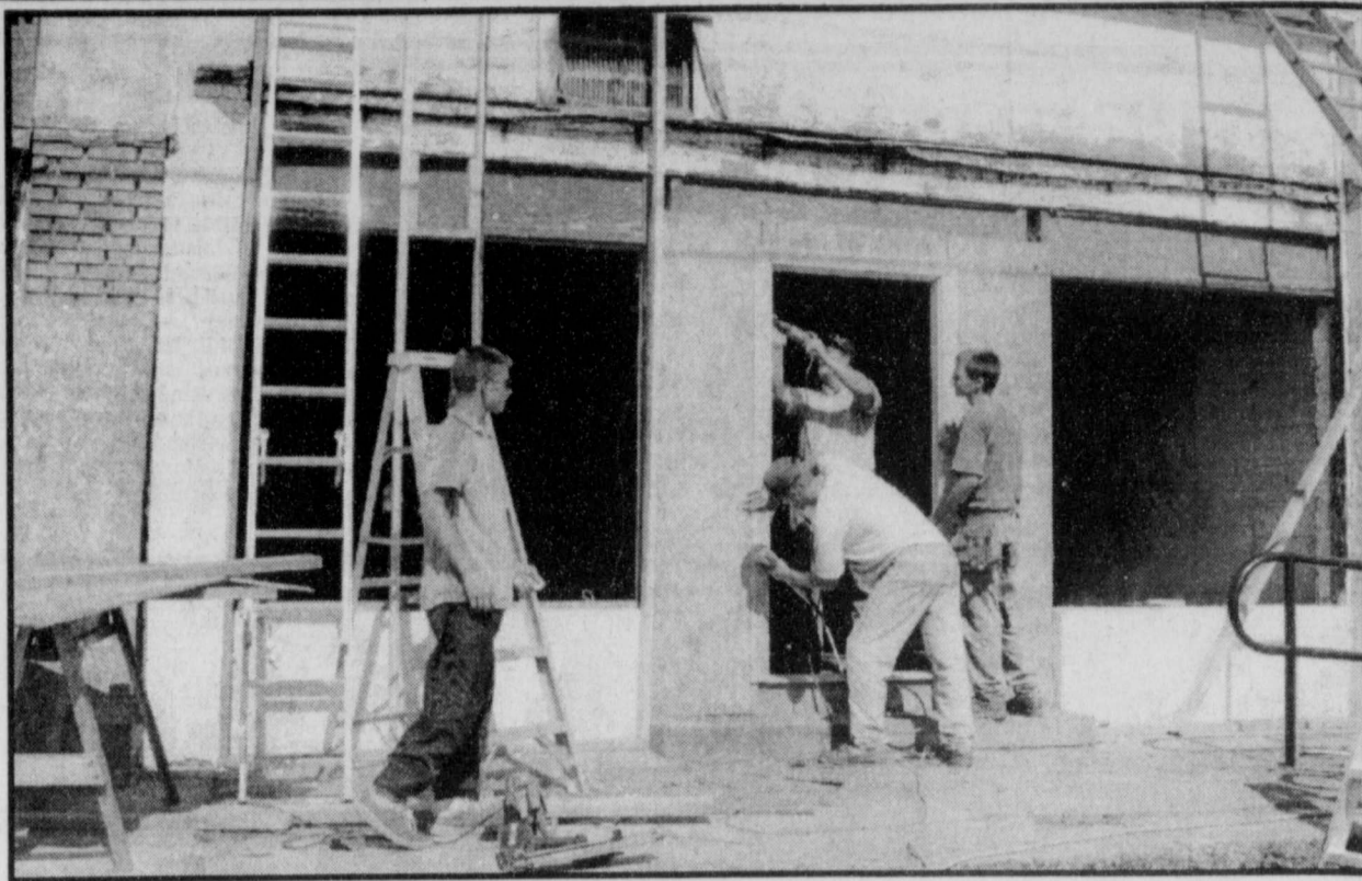
WORK -David Ham, Joey Ham, Daniel Ham and Sammy Ham worked on replacing the store front on the old hardware building on the north end of Main Street in Deport last Monday. Ham says his plans are to open a recording studio in the building sometime in the future. (Staff Photo by Thomas Nichols)
