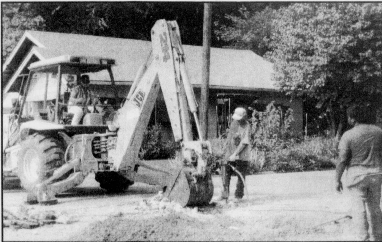
SUPT. Gary Reed, Scott Wooten and Chester Taylor, all of Pioneer Mechanical Contractors, Inc. of Texarkana dug a hole in Monroe Street in Deport Monday as they begin a project. New sewer lines, water lines and fire hydrants will be installed on part of Depot Street, Church Street and College Street. (Staff Photo by Thomas Nichols)
