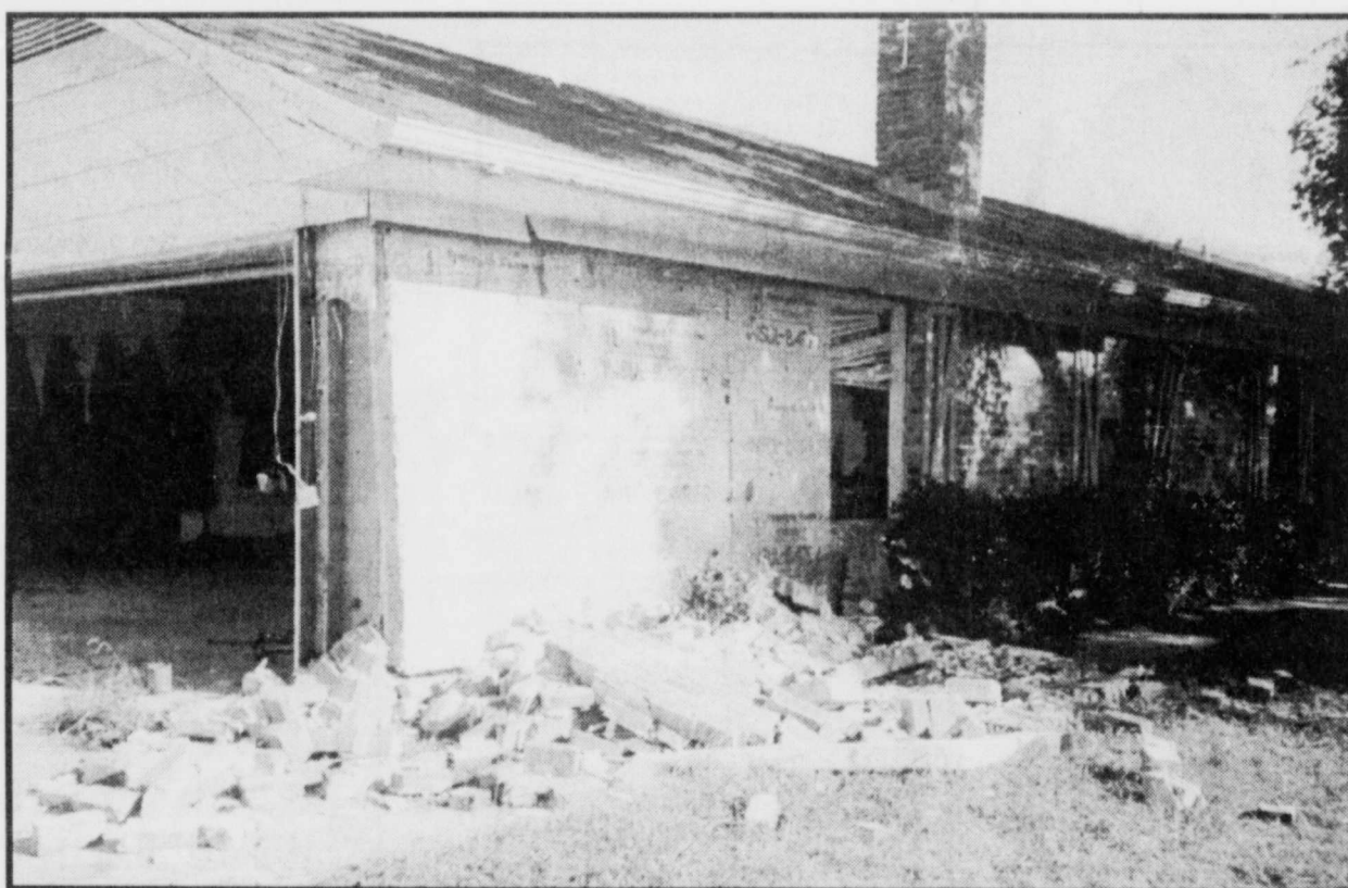
HEAVY DAMAGE-the home of Danny and Callie Gaddy sustained damage to the brick and windows, plus the tornado lifted the roof so that wall damage inside occurred. The tornado occurred Friday night, in the Pattonville area, as did golf ball size hail, high winds and heavy rain. (Staff Photo by Barbara McDowra)
