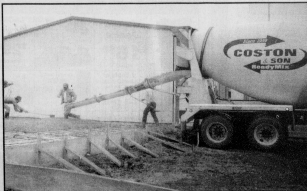
POURING CONCRETE-work has begun on the new addition to the Pattonville Fire Station and Community Center with the pouring of a concrete slab for their new bay. (Staff Photo by Barbara McDowra)
