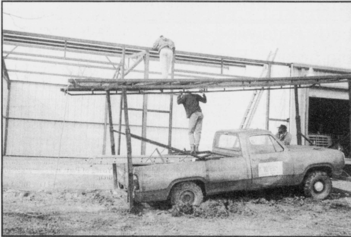
DONALD DAY and helper are working putting up the frame work for the new addition to the Pattonville Community Center/Fire Department. It is hoped the next dance will be held on the new area! (Staff Photo by Barbara McDowra)
