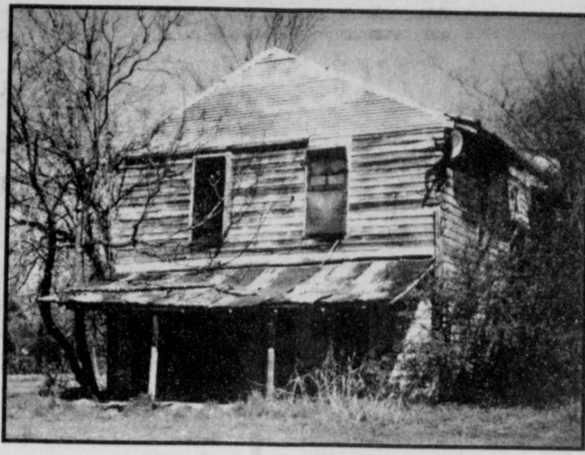
Only a deserted building now, Taylor Town store was once the center of a thriving community
