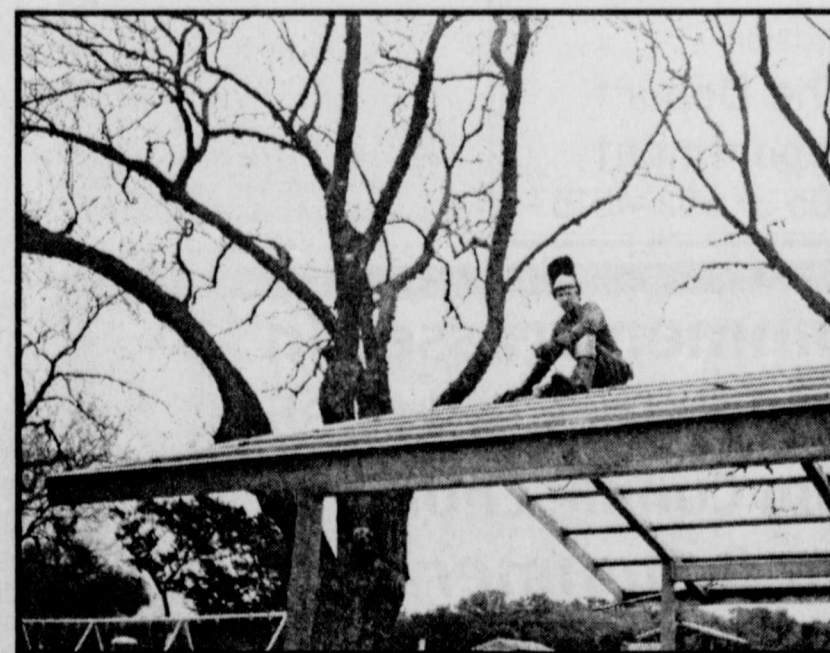
WELDING FOR LBJ- Thomas Crossland of Pattonville was recently worked on construction of picnic tables and covers on the LBJ ranch recently.
