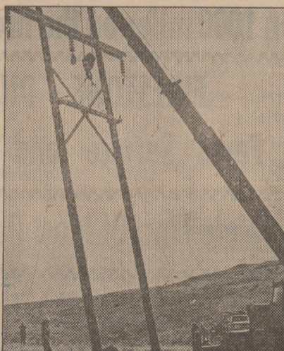
"We're putting in a new 115,000 volt line . . . gives us another feed to back up our dependability . . ."
