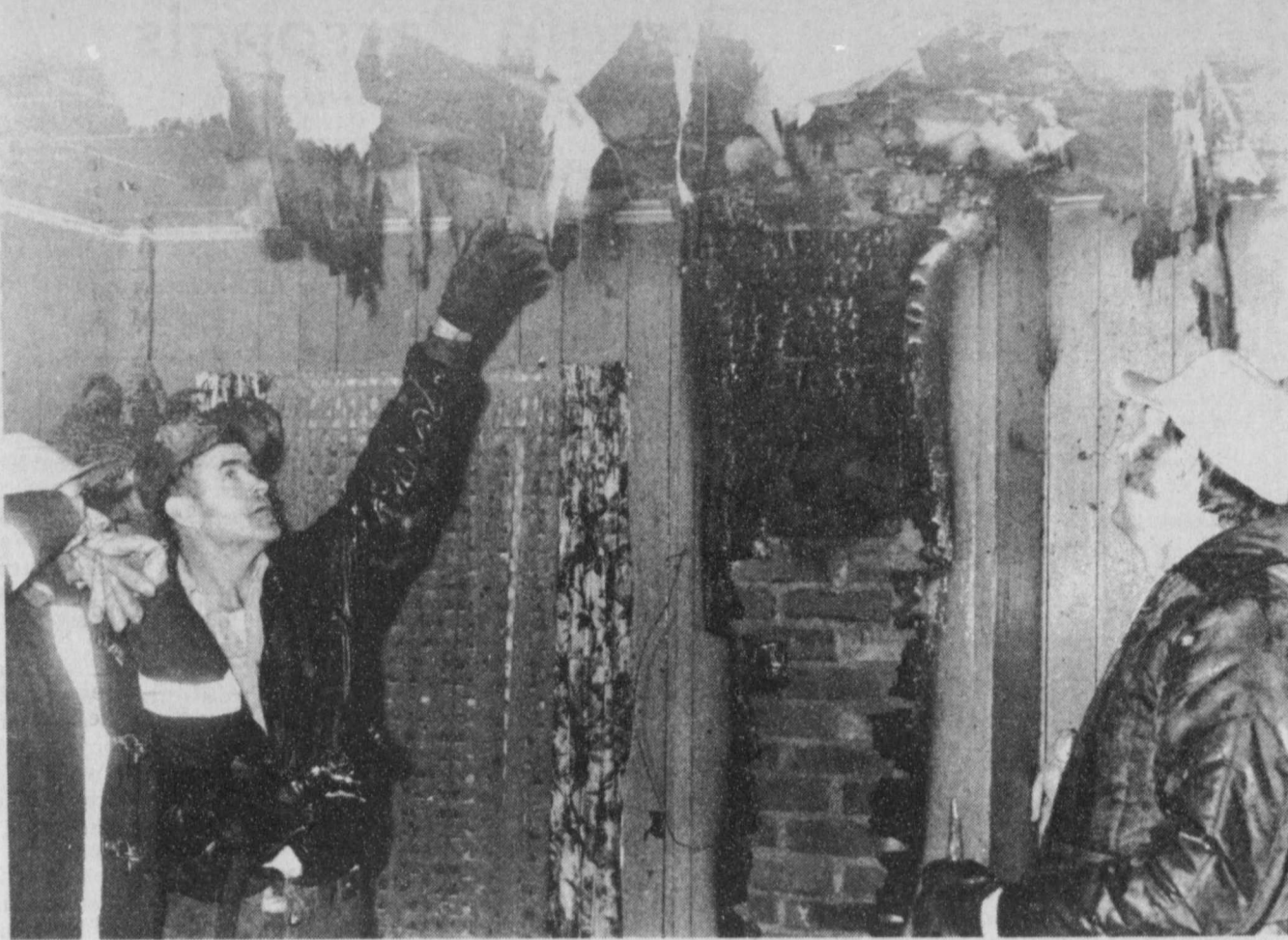
PATTONVILLE Volunteer Fire Department had already extinguished the fire at the home of Bob and Stella George between Pattonville and Deport when
