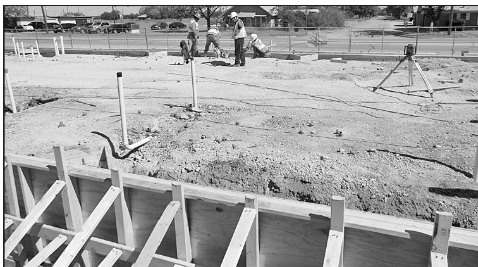
NEW CONCRETE —Workers are preparing to pour the footings for the new Emergency Room building at Haskell Memorial Hospital.
