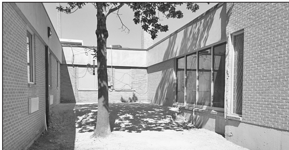
LAB EXPANSION —Dirt work is being done to prepare for the expansion of the lab at Haskell Memorial Hospital. The new wall will be east of the existing structure in the courtyard area.
