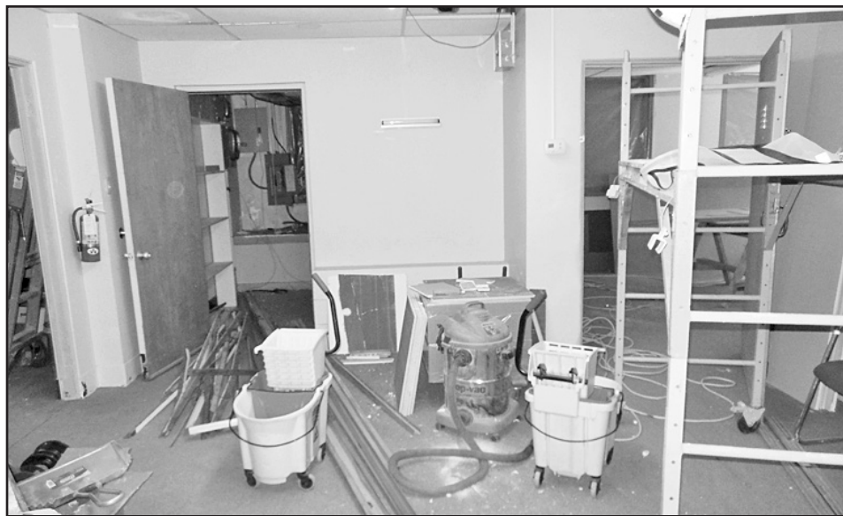
HOSPITAL PROJECT —Progress is being made on the improvements underway at Haskell Memorial Hospital. This area is being readied for the location of the new entrance to the Emergency Room.
