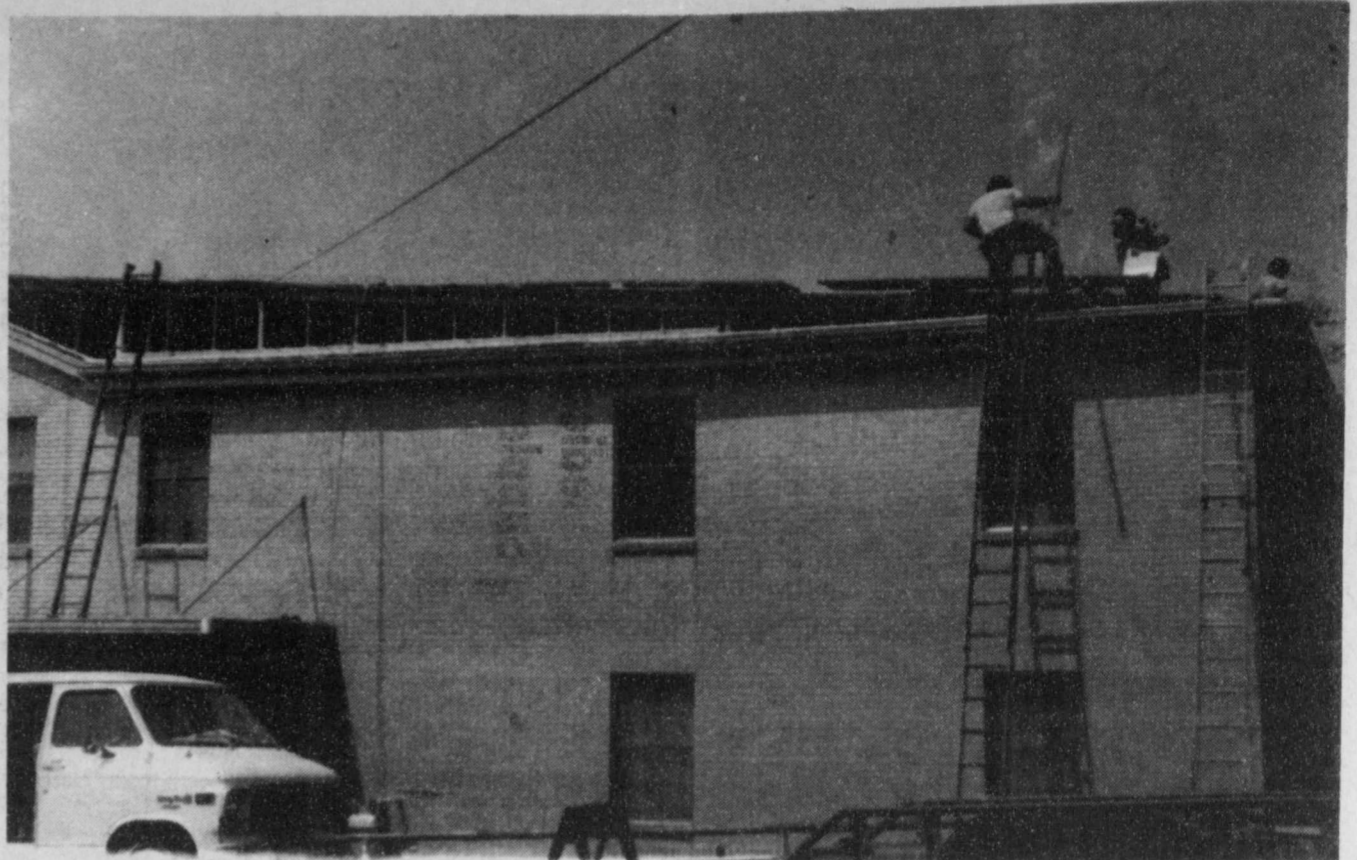
NEW ROOF—The First Baptist Church of Bogata is receiving a new roof at present. The old, flat,
