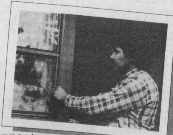
TNP Employee Ruben Reyes uses inexpensive caulk and weatherstripping to seal in indoor comfort... and you can too!
