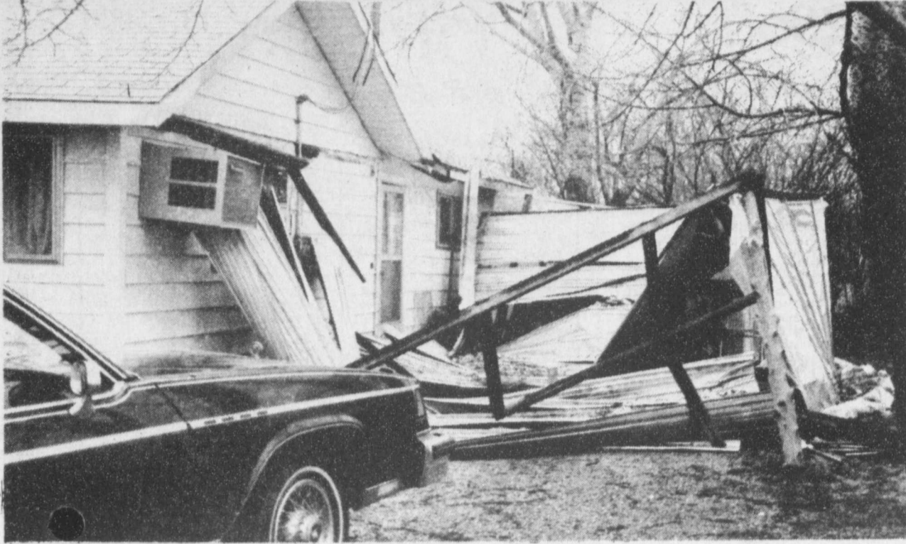
THE CARPORT at the home of Mr. and Mrs. Cliff Jones collapsed from the heavy load of hail that hit Talco Wednesday afternoon. (Staff Photo)
