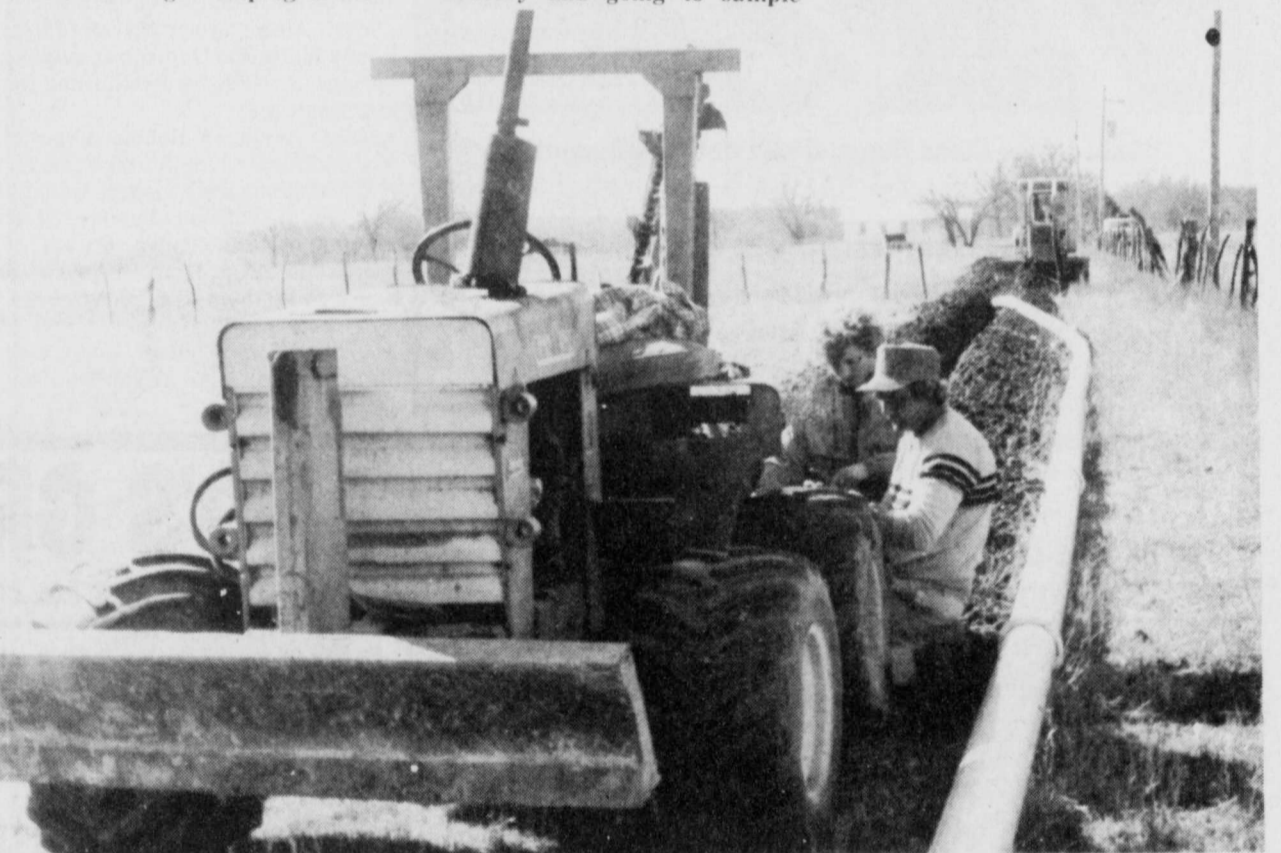
WATER LINE for Red River County. A Louisiana Construction Company has been busy laying a six-inch water line across Hwy. 271 to Fulbright. It will tie off and an eight-inch line will come to the Lamar County Water tower at
