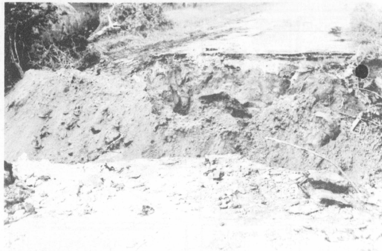
BRIDGE OUT —There is no bridge on 3rd St. N.E. close to the com-
