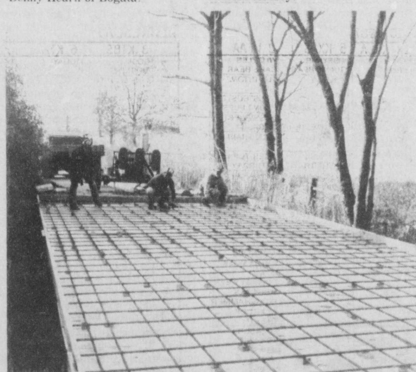
COUNTY WORKERS were busy Monday, December 29, replacing the old bridge south of Bogata, which runs into Highway 271, with a new concrete bridge. The new bridge is one of several which
