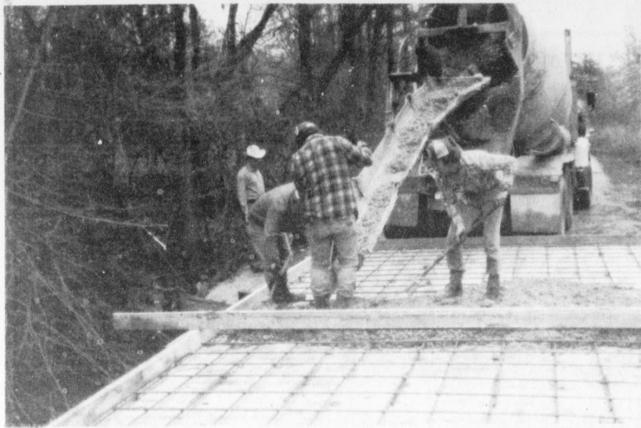
THE BRIDGE on the Pine Branch road is being replaced with a concrete one. County workers started the work last week. According to Precinct 1 County Commissioner, Drue Pirtle, the bridge should be finished this week. (Staff Photo)
