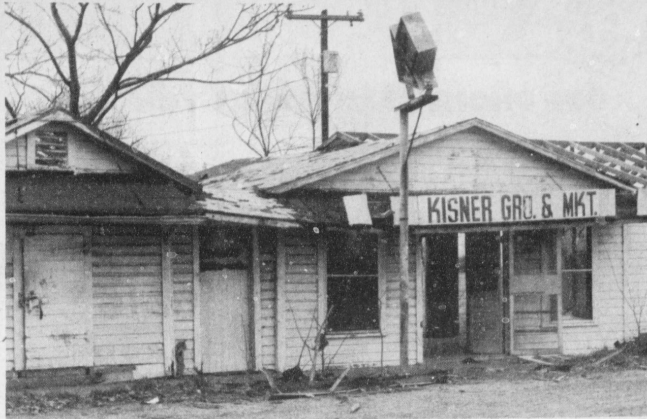
WORKERS began last week tearing down the building which was Kisner's Grocery Store. The
