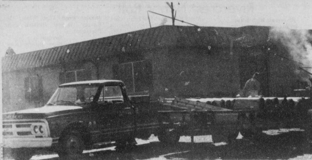
NEW ROOF-Red River Haven Nursing Home in Bogata is getting a complete new roof. The work is being done by Garcia Roofing Co. from south Texas. (Staff Photo by Moille Williams)
