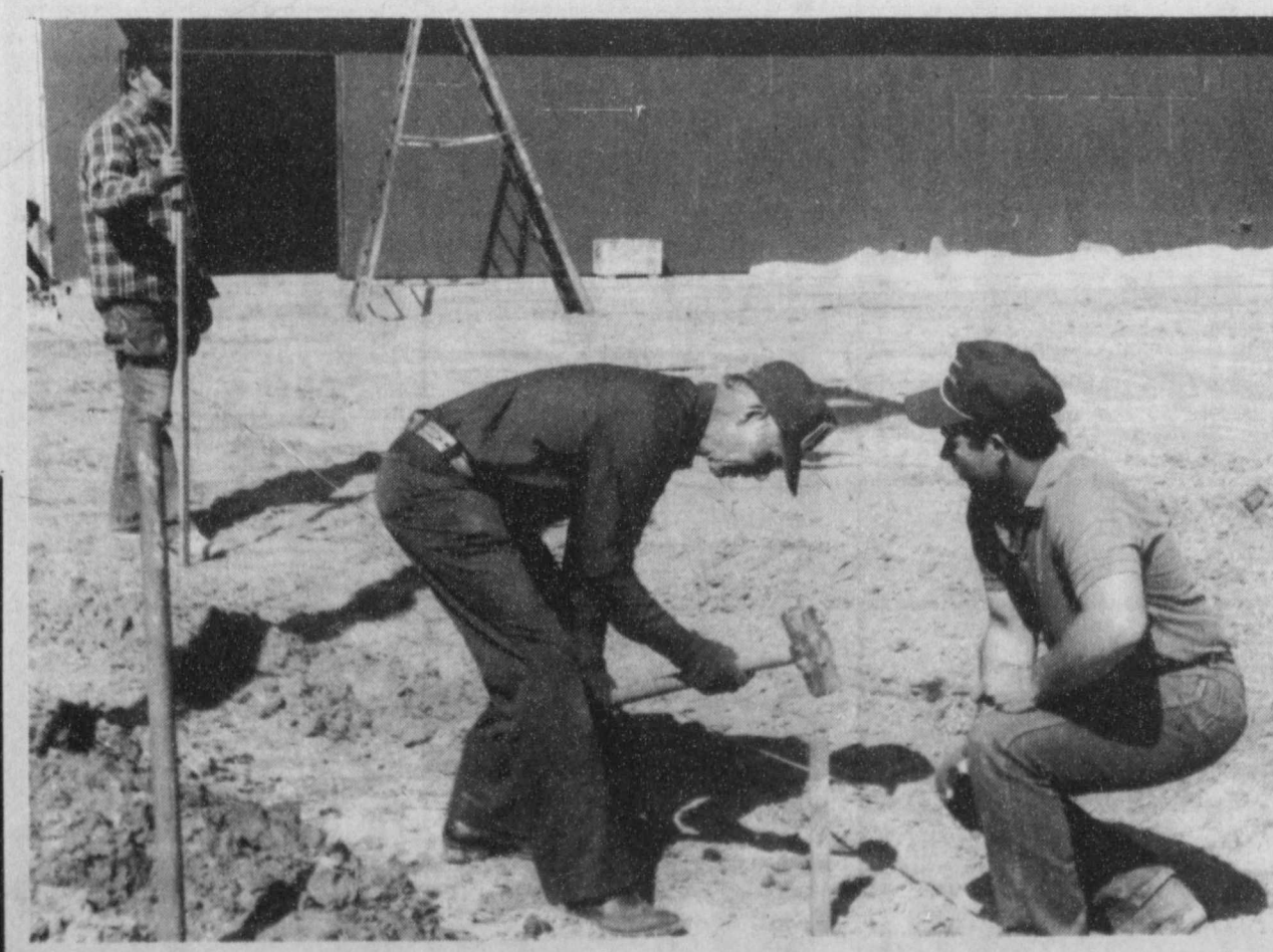
NEW STORE-Workers are busy at the new grocery store going up in Talco. (Staff Photo)
