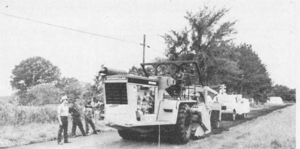
RECLAIMER-This giant Caterpillar RR-250 was demonstrated at Jolntown last Thursday. The machine is called a reclaimer, it tills down four inches, mixes and breaks down the existing oil pavement and leaves an improved surface. (Staff Photo by Mollie Williams)
