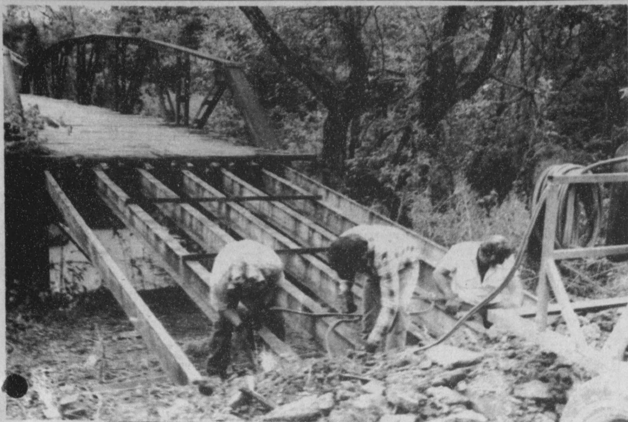
ROADCREWS from Red River and Titus Counties were busy Wednesday, October 5, tearing out each end of the bridge across Sulphur River in preparation for repairs. (Staff Photo by Mollie Williams)
