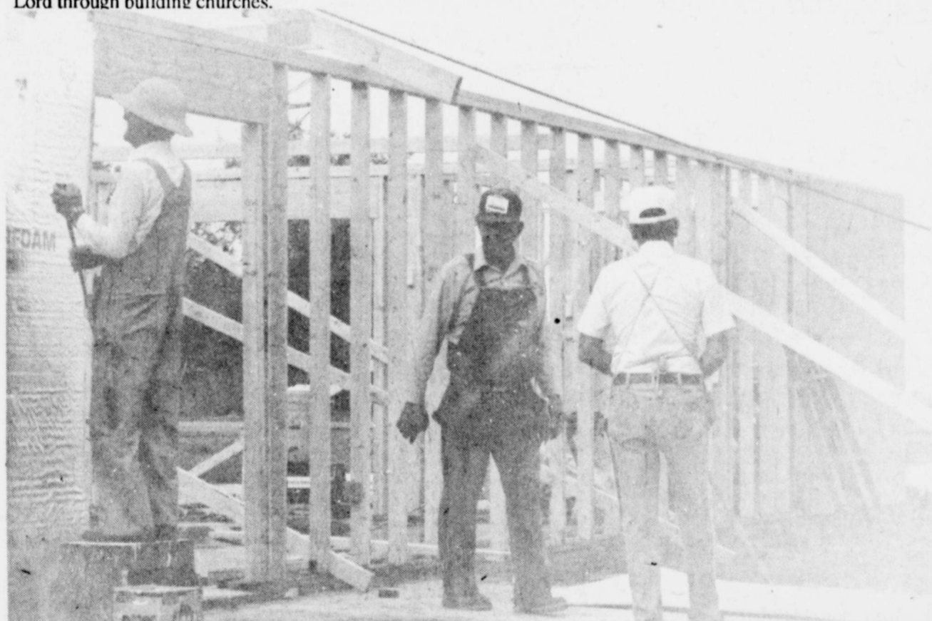
GOING UP -Twenty three retired Baptist men were on hand Monday morning to begin building the Cunningham Baptist Church. The group travels all over the state and beyond erecting churches, and the only pay they ask for is one meal a day. The men and their wives camp in camping trailers on site, and
