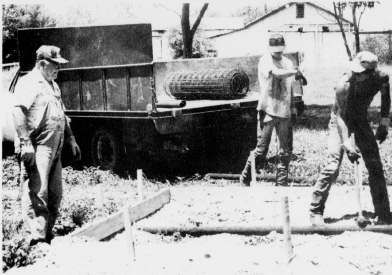
HARD AT Work , in spite of the heat. These men were busy preparing to pour concrete for picnic tables at the Talco Community Park., Inc. From left to
