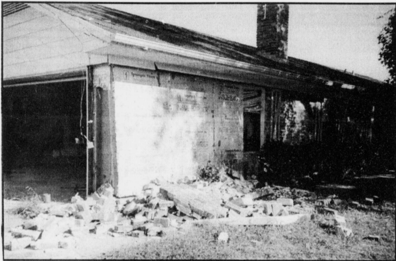
HEAVY DAMAGE -the home of Danny and Callie Gaddy sustained damage to the brick and windows, plus the tornado lifted the roof so that wall damage inside occurred. The tornado occurred Friday night, in the Pattonville area, as did golf ball size hail, high winds and heavy rain. (Staff Photo by Barbara McDowra)
