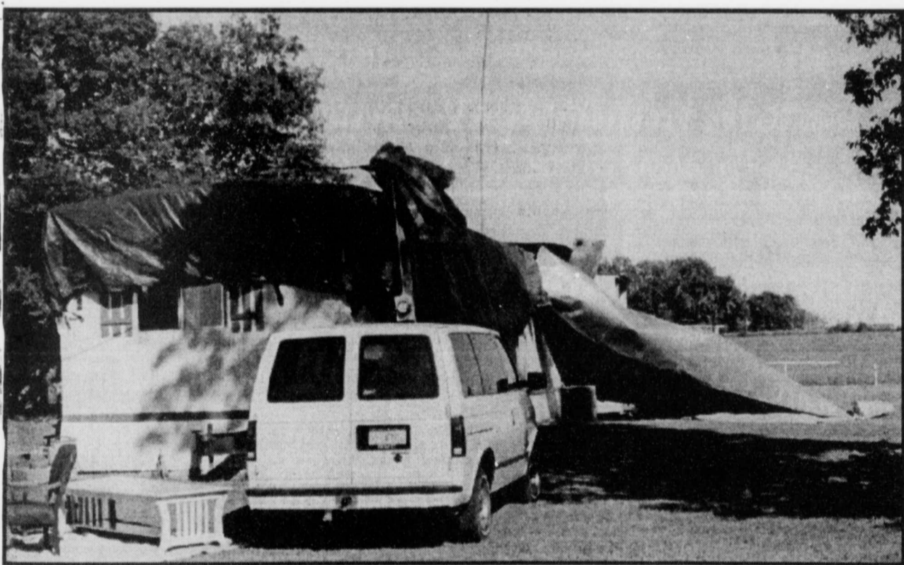
ROOFLESS -the mobile home of the Joe Barrentine family was ripped loose and their possessions soaked last Friday night when a huge storm swept through the area. The Barrentines report that they saw the tornado which did the damage. They report that the suction from the funnel did the damage, and that the actual twister missed their home. They are living in camper trailers until they can build back. Nearby round bales of hay were blown across the road, and golf ball size hail also fell. (Staff Photo by Nanalee Nichols)
